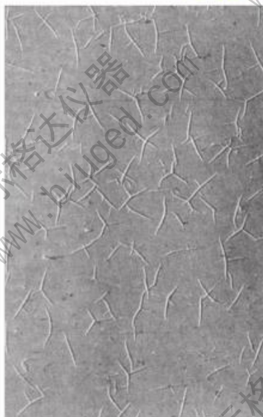
Figure 5 — Crow's foot cracking
